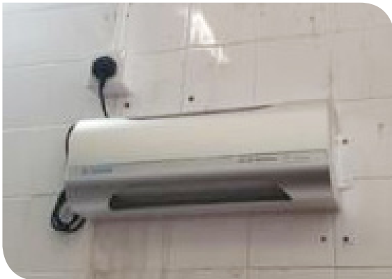
UV air sterilisation device for garbage room – Mount Regalia
