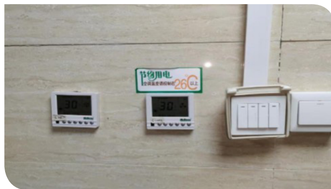
Signs placed in the hotel lobbies and guestrooms in Regal Airport Hotel, Xi'an to remind employees and guests to turn off electronic appliances after use to save energy
