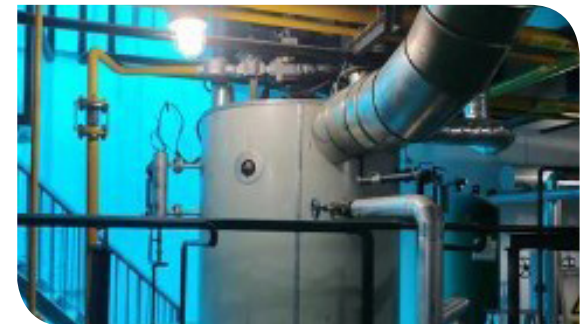
Boilers are renewed with more energy efficient models and achieved 8% of energy saving in Regal Airport Hotel, Xi'an.
