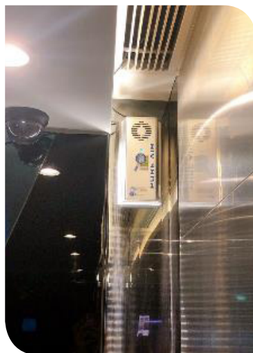
UV air purifiers in the lift
